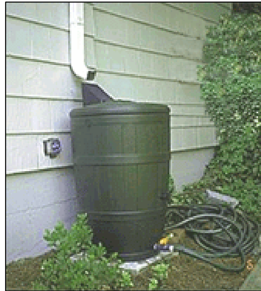
Figure 4-25. A typical rain barrel set-up at a residence. (Source: Low Impact Development Center)
