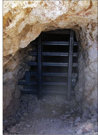
Following the design workshop, four abandoned mines were secured and a bat gate was installed at one adit with evidence of bat activity.
